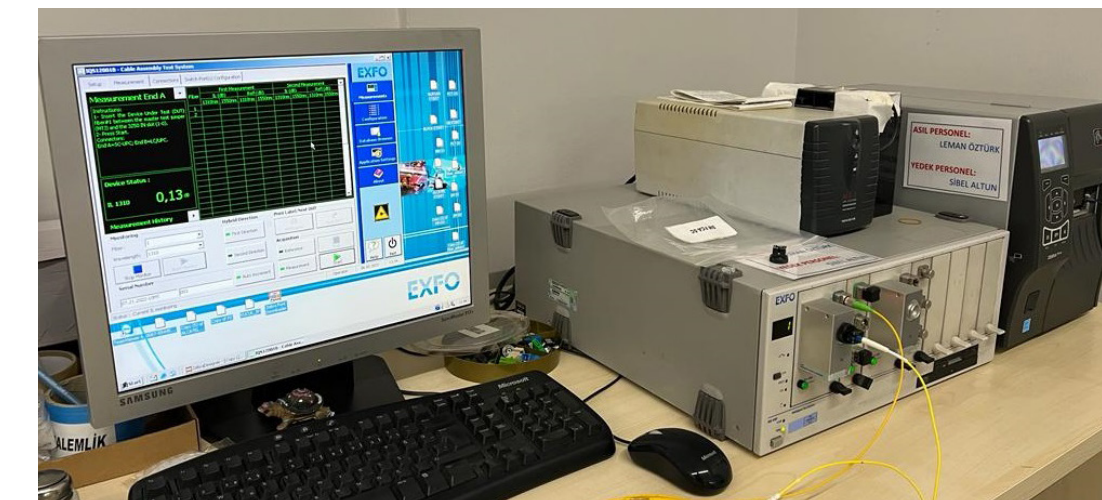
• Fiber Optic Digital Test
